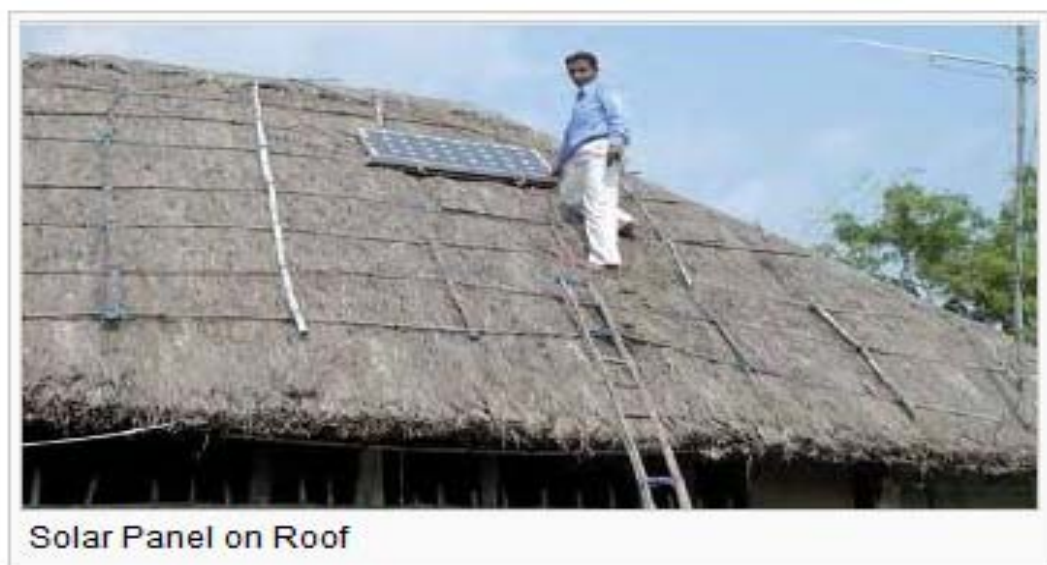
Figure 3.Solar panel on the roof.
