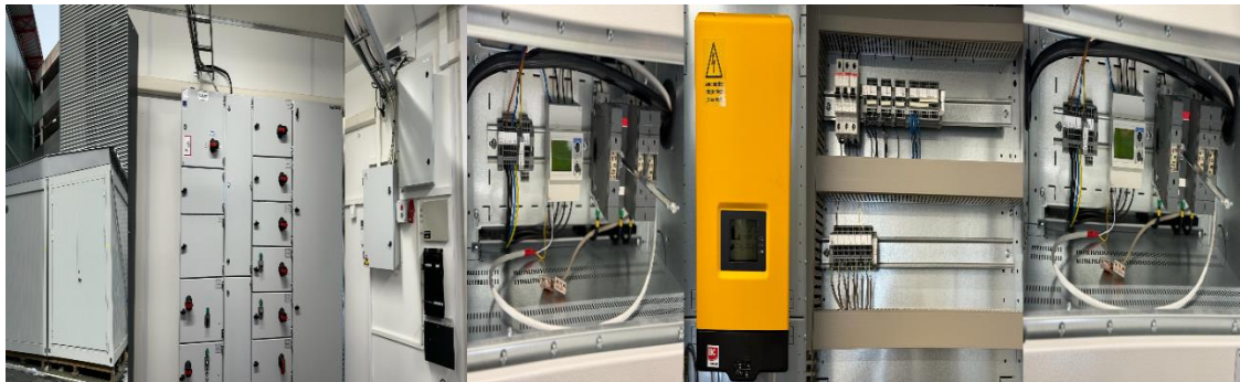
Figure 1. Solar plant system at Savonia UAS
