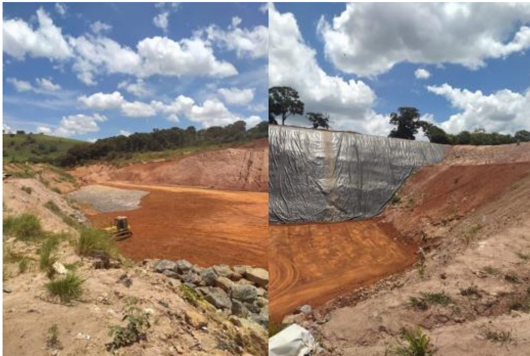
Figure 17 - Waterproofed landfill areas for receiving waste in Pouso Alegre
