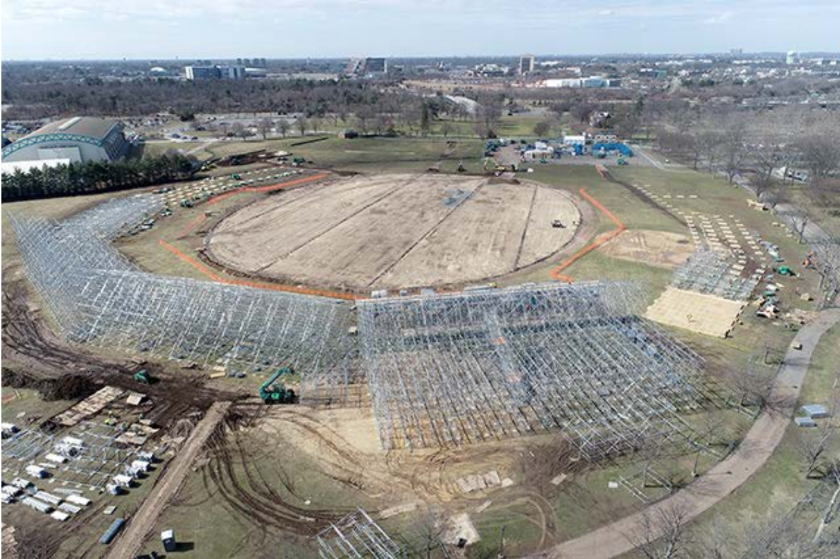
Figure 35: Construction in progress for the stadium site in Eisenhower Park in March 2024
