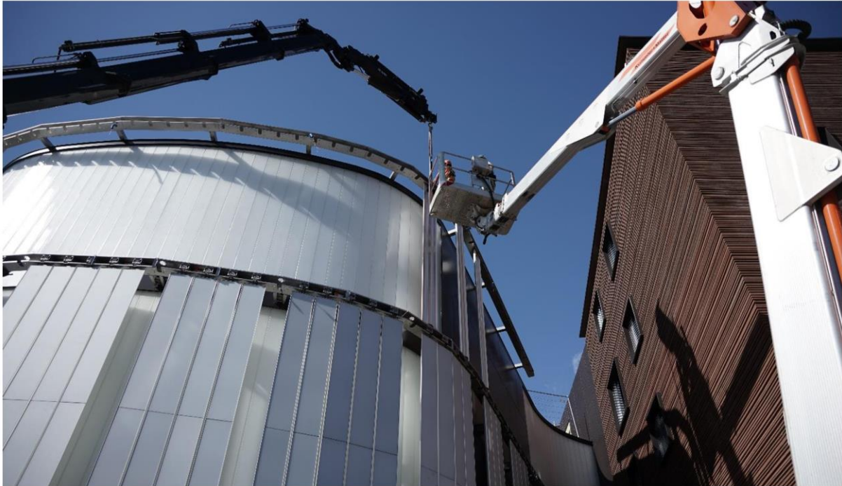
Fig. 18: An image showing the installation of the BIPV slats (Corti, et al., 2022)
