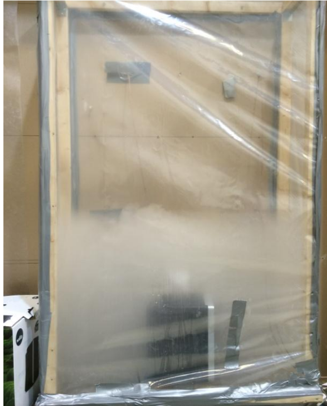
Figure 25 Wall installed with humidifier
