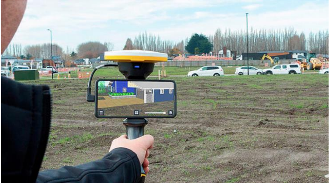
PICTURE 6. You can see the IFC model shown in the location where the future building is designed (Geotrim 2024).
