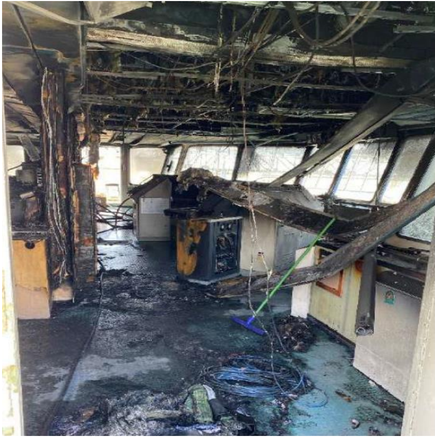
Figure 3. Damage of fire to the bridge. (NTSB, 2023).
