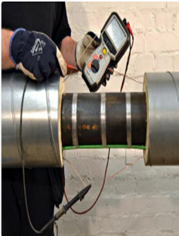
PICTURE 7. Resistance measurement of alarm wire loop (Jari Randell)
