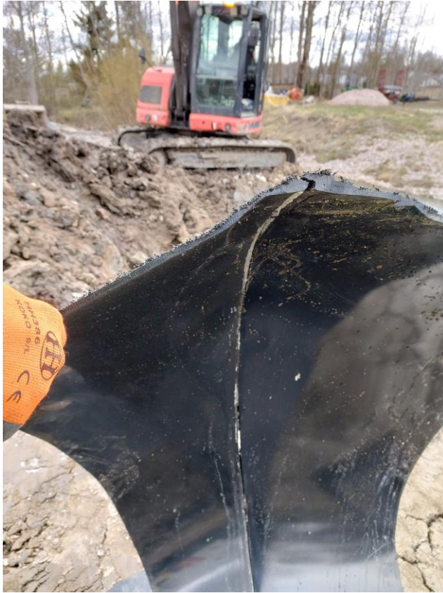
PICTURE 15. Broken protective sheath joint (Jari Randell)
