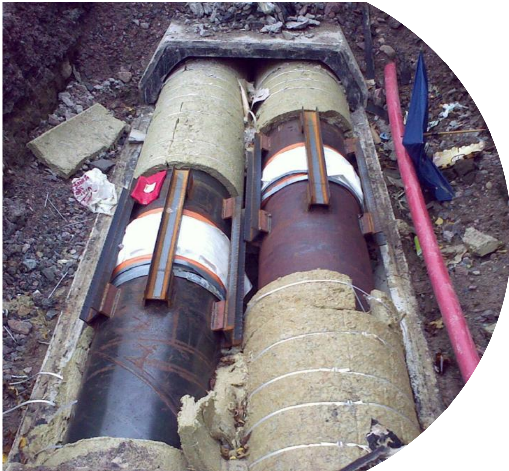
PICTURE 3. Concrete duct district heating line (Henrikki Nuutinen, Helen Oy)
