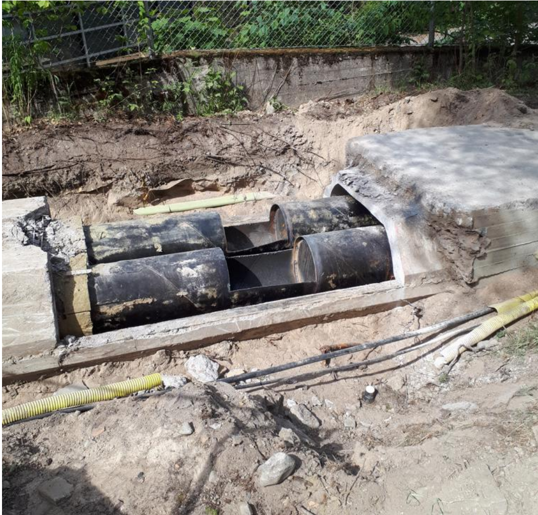
PICTURE 2. Concrete duct district heating line (Jari Randell)
