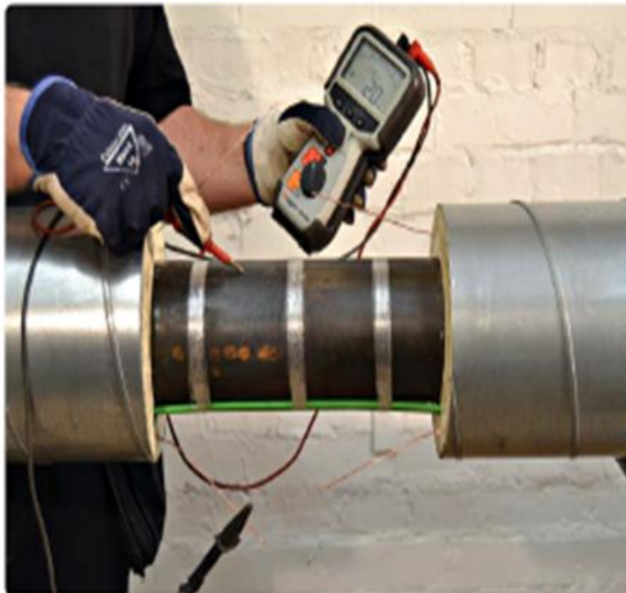
PICTURE 8. Resistance measurement between alarm wire and flow pipe (Jari Randell)
