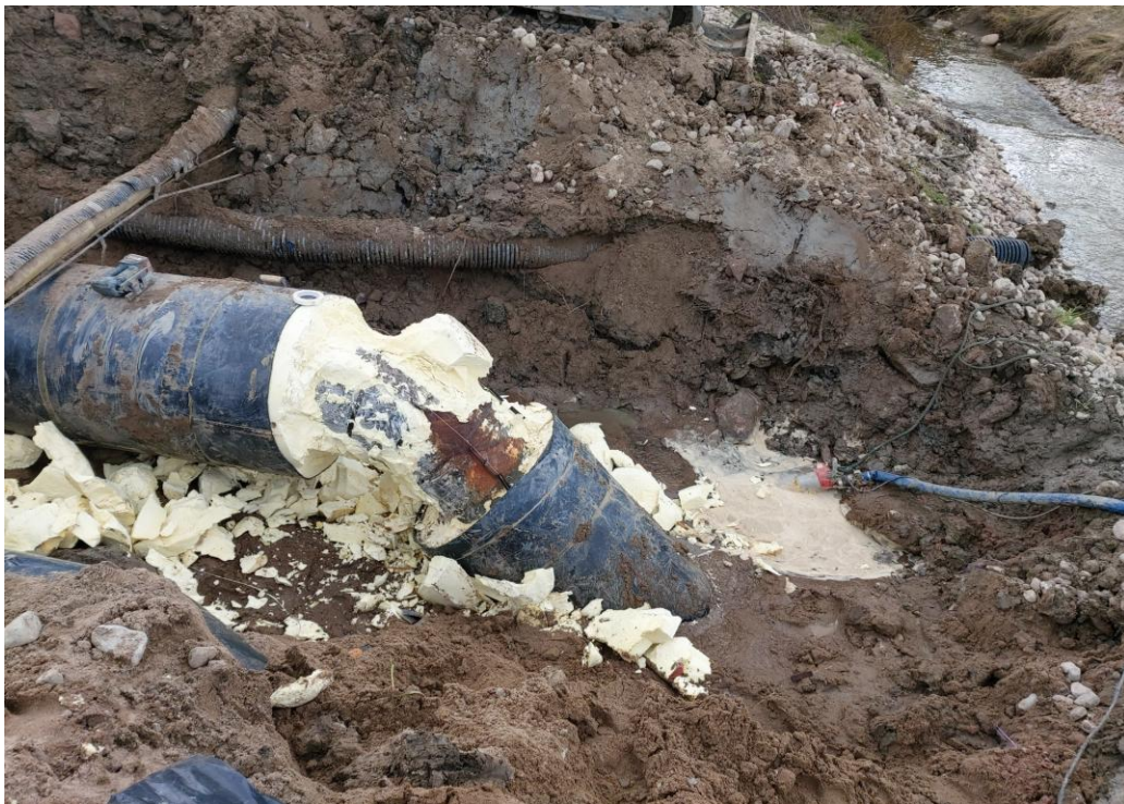
PICTURE 16. Corroded flow pipe (Jari Randell)
