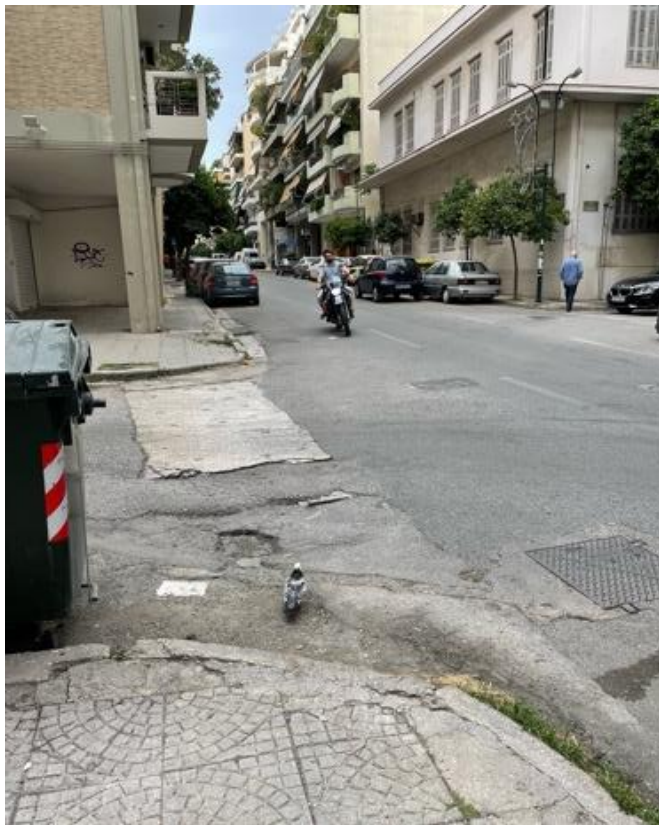
Photo 3. A destroyed ramp at a neighborhood.
