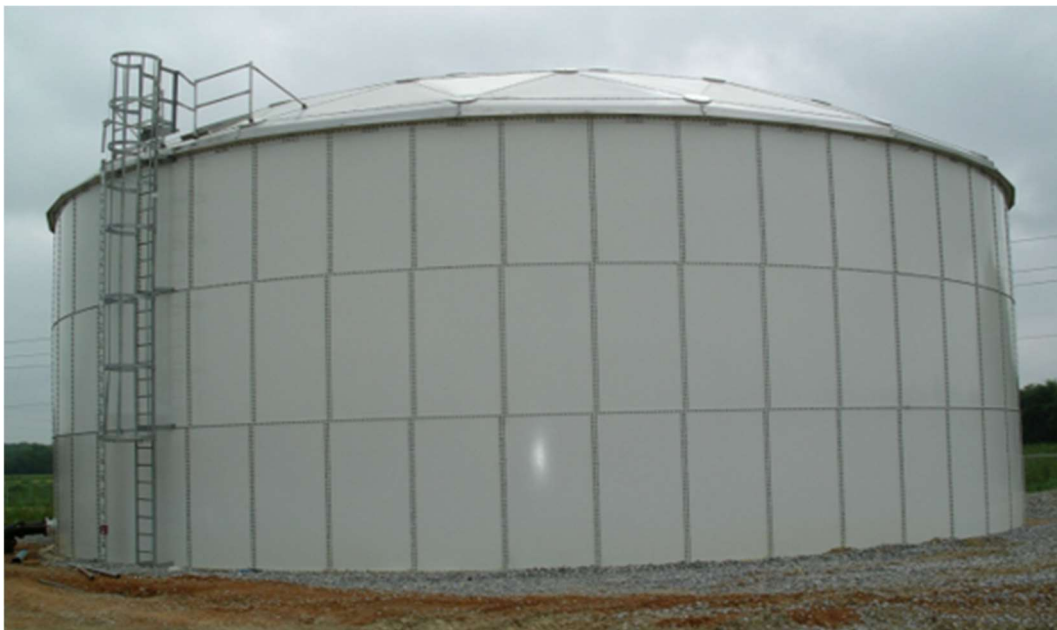
Figure 9. Bolted tank (Steven Brown & Associates Inc, 2025)
