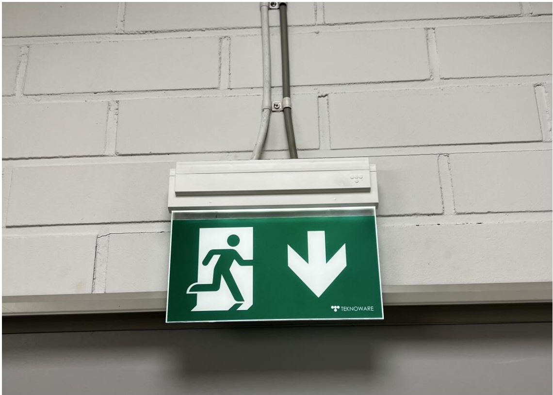
Figure 1. Maintained emergency luminaire installed atop a door.
