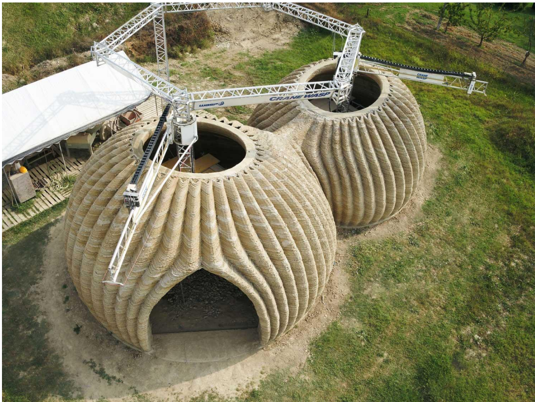
Figure 13: TECLA printed structures (Copyright © Mario Cucinella Architects and WASP, 2021). Photo by Iago Corazza..
