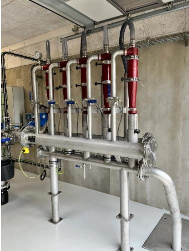
Figure 1 Hydrocyclone station at Søholt WWTP
