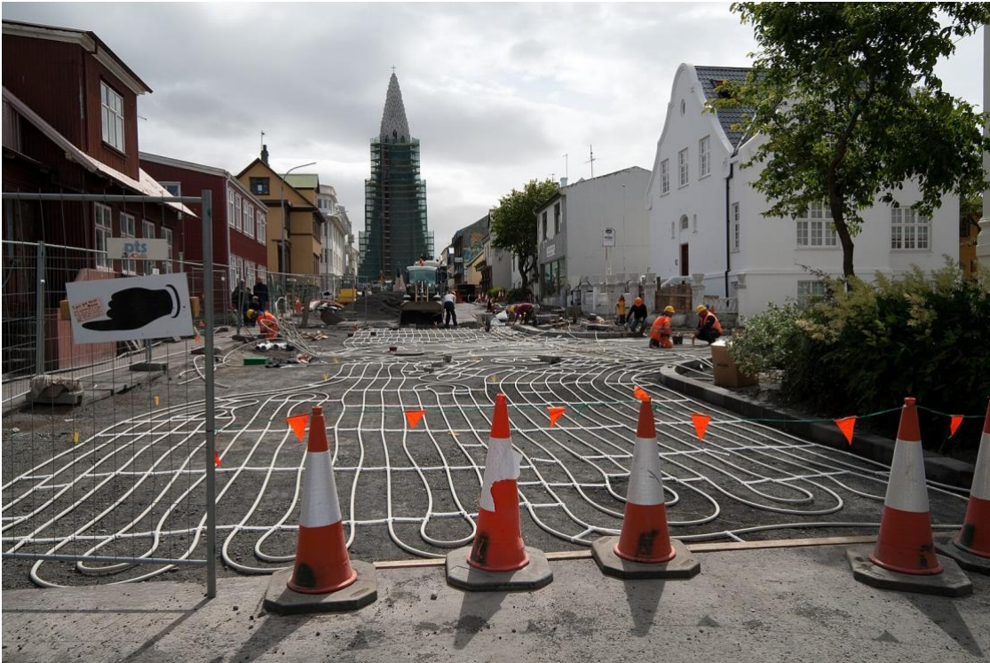
Figure 8. Installation of a geothermal snowmelt system on a street in Reykjavík, Iceland [22]
