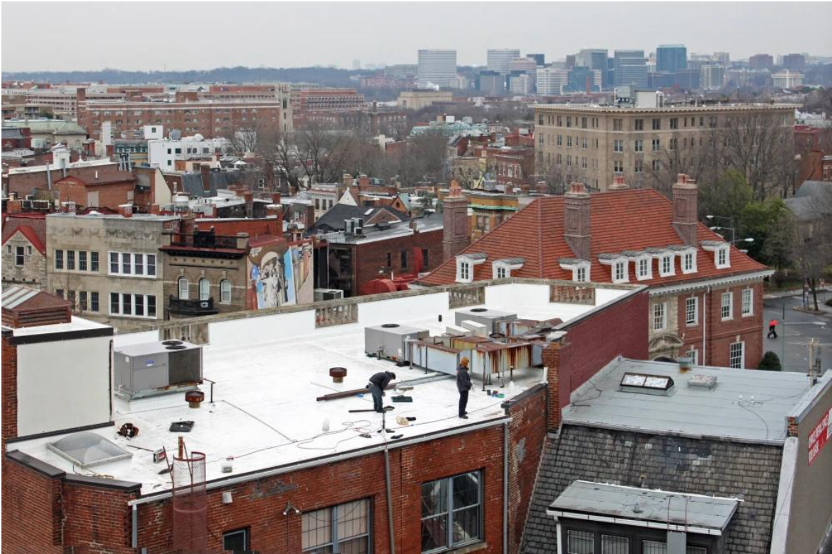
Figure 5. A construction crew paints a white roof in downtown Washington, D.C. (María-José Viñas 2010)
