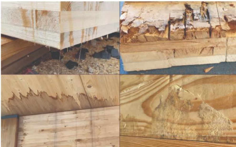
Figure 16. Moisture damage in CLT (Vaproshield, 2020)
