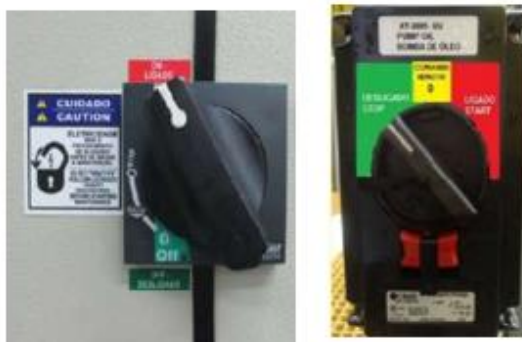
Figure 10. Main Switch color for compliance.
