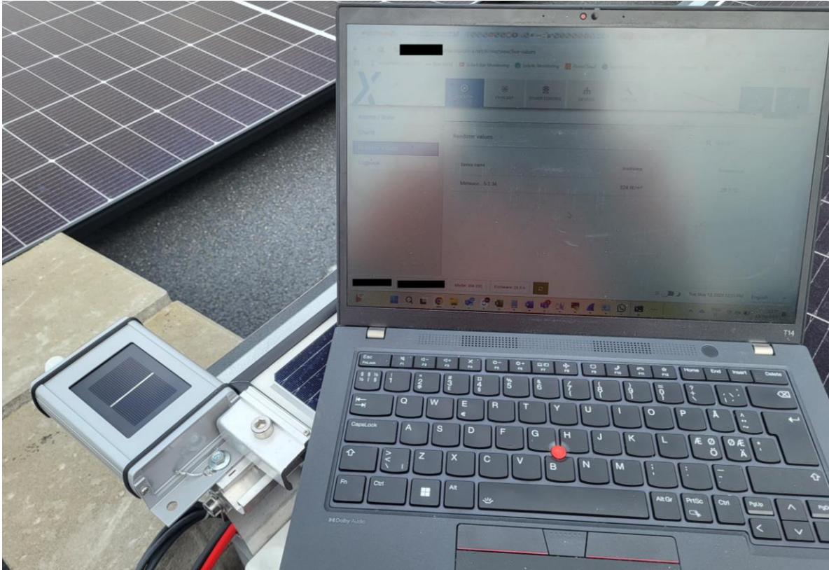
Figure 9 Irradiance sensor installation and testing of the sensor via VCOM (Photograph by the author, 2025)
