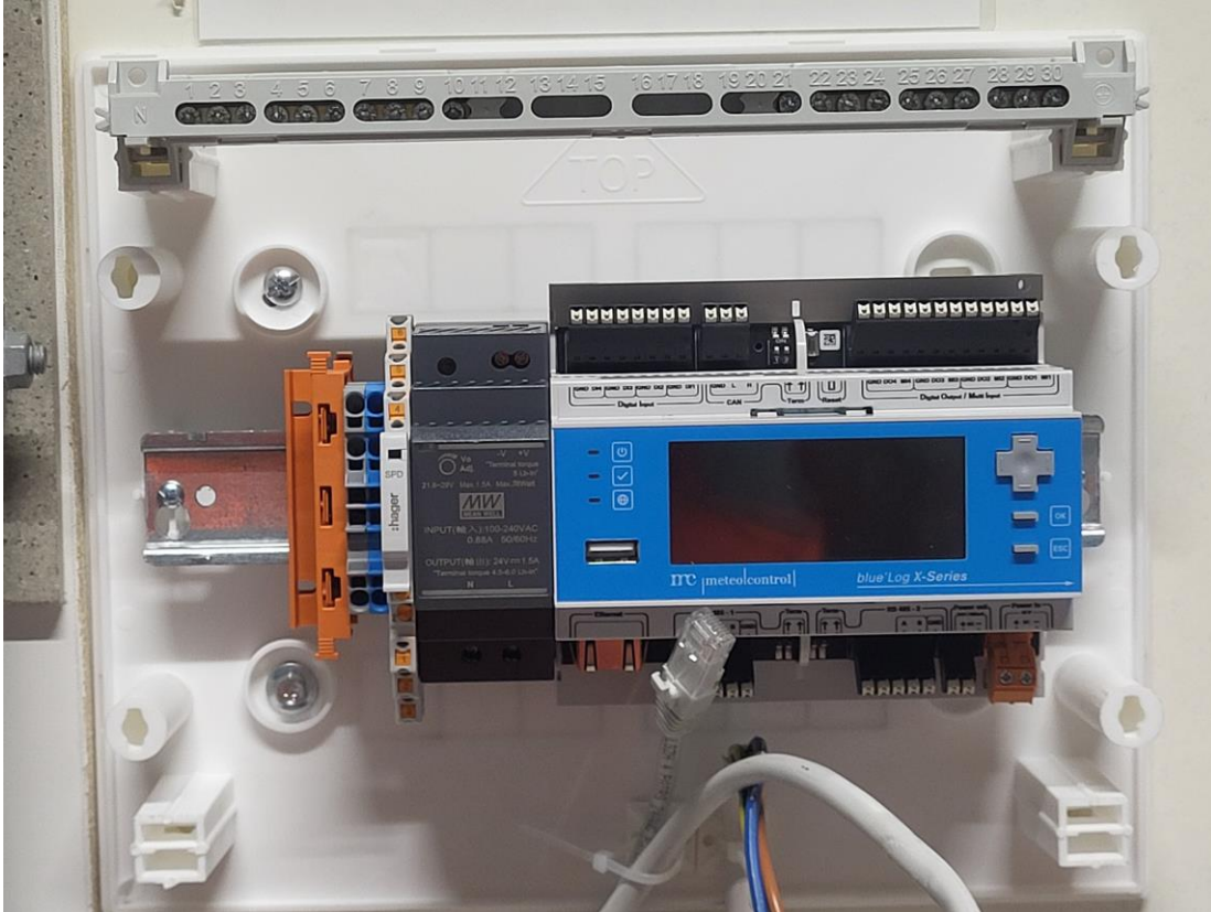
Figure 6 The enclosure with the devices installed (Photograph by the author, 2025)
