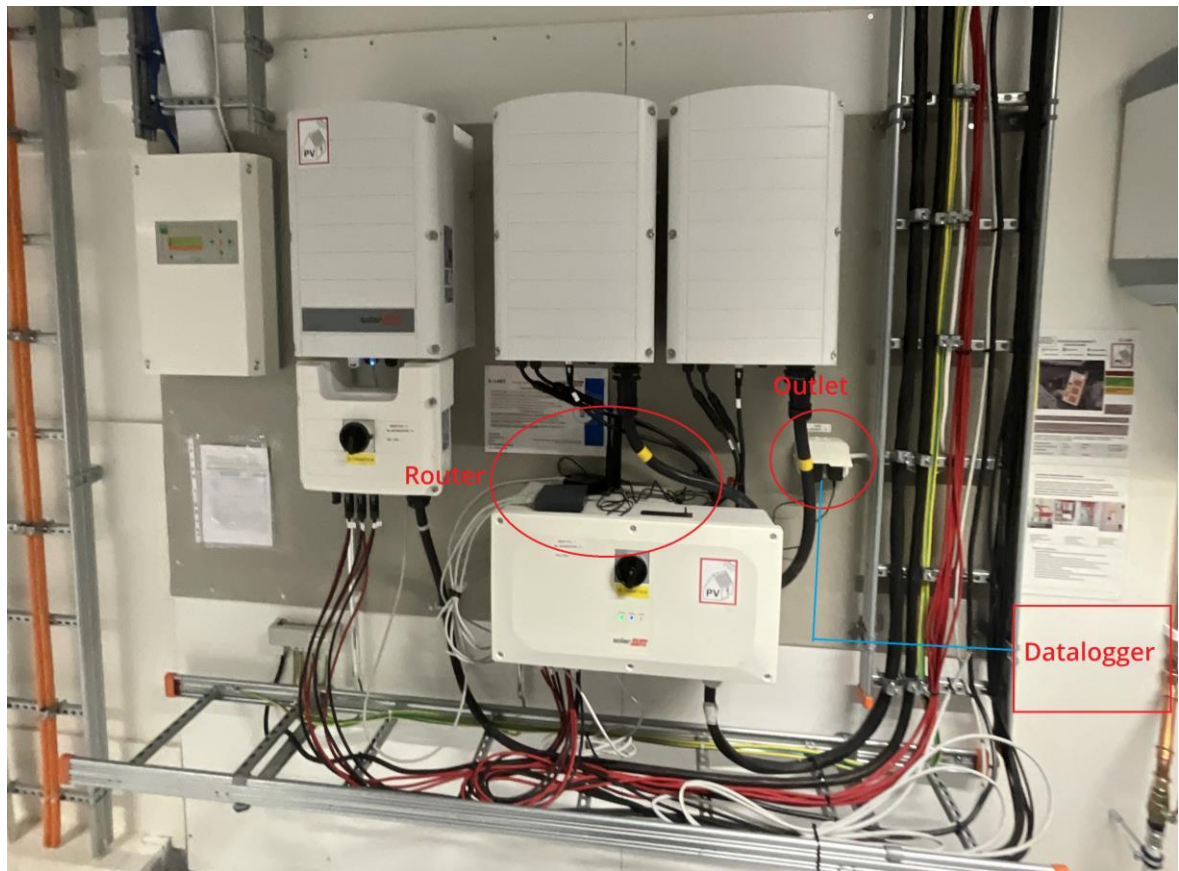
Figure 5 Location of the components in the system (Photograph by the author, 2025)
