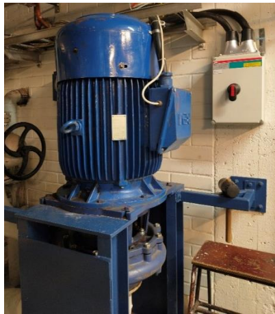
Figure 23. The 55 kW Induction Pump at the Åland Energy Laboratory
