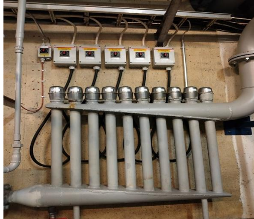
Figure 25. Resistive heater units at the Åland Energy Laboratory
