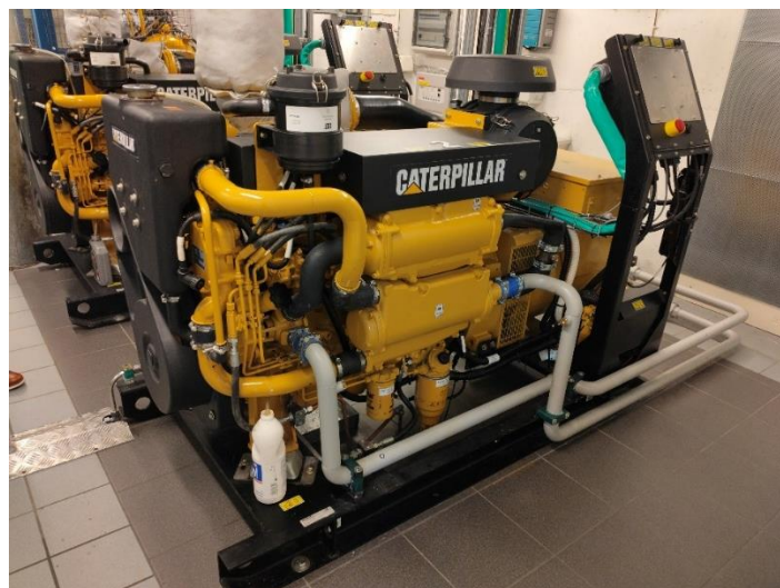
Figure 14. CAT C6.6 Diesel Generators at the Åland Energy Laboratory
