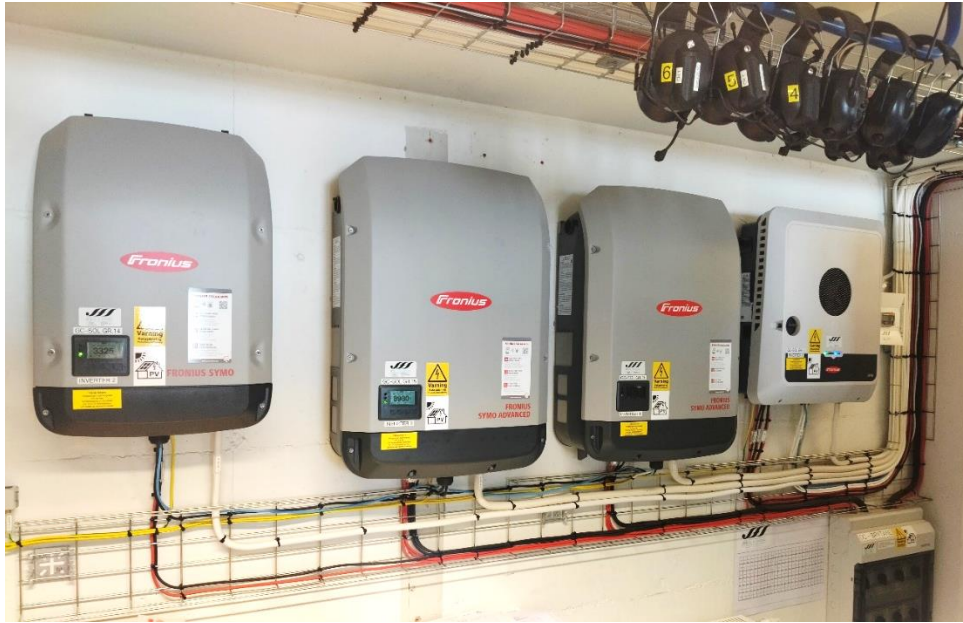
Figure 13. Solar inverters and battery energy storage system (BESS) setup at the Åland Energy Laboratory.
