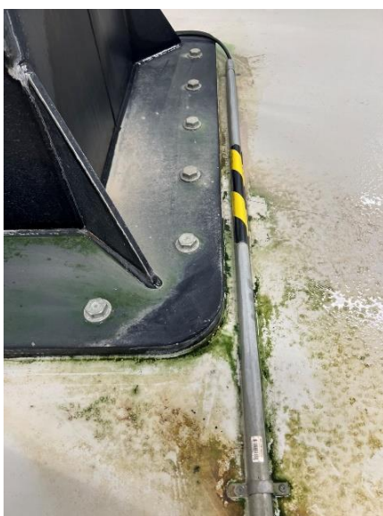
Figure 9. Residual water and contamination on the floor due to splashing from the current open washing system.
