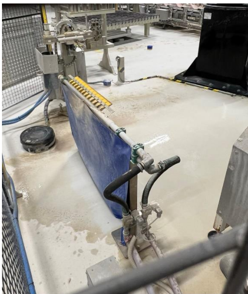
Figure 2. Washing area after operation with current open setup. The floor remains wet with visible puddles.
