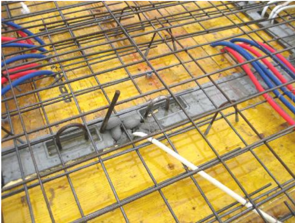
Img. 504. There are hooks in the top of the load bearing element wall. They are only for be able to hoist the element. The connexion of these wall elements to the cast concrete is provided by the vertical steel bars. These bars also later will be the connexion with the wall element above.
