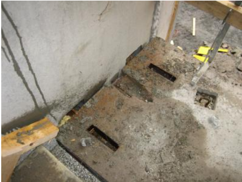
Img. 387. Intermediate slab placed, hold by the sliding steel supports to the walls
