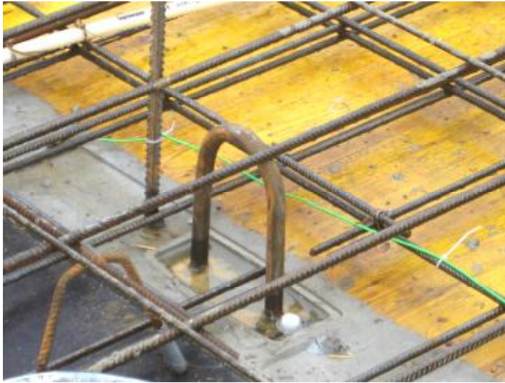
Img. 517. Detail of the temperature gauge system cable for measuring the temperature of the fresh concrete
