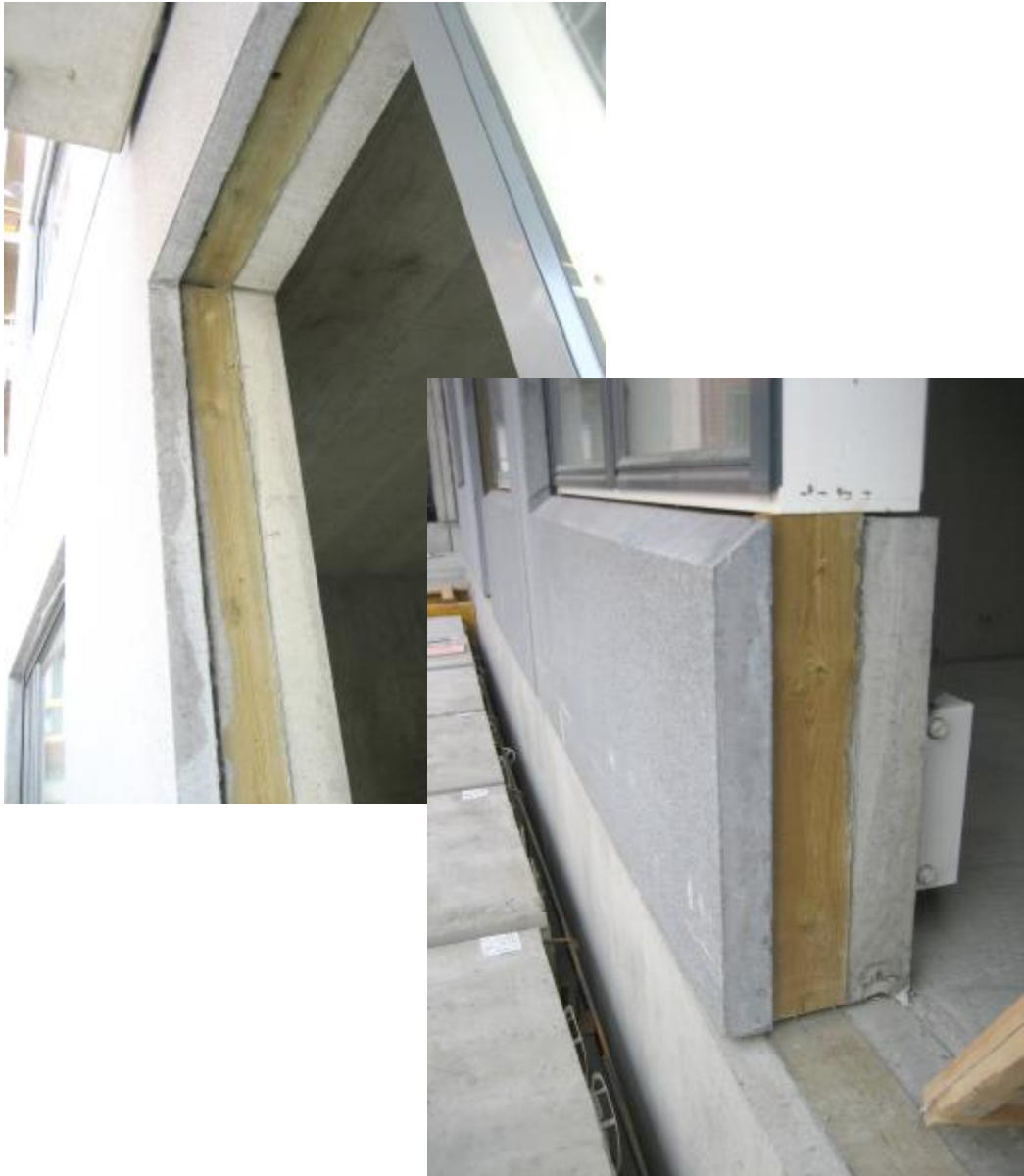
Img. 327, 328. Detail of the wood frame, which fulfills the double function to close the hollow of insulating material in the perimeter of the hollows in the panel, and of using as support for the carpentry that will be screwed into it.
