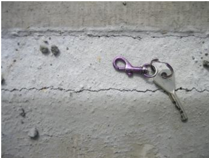
Img. 352. Detail of retraction fissure
