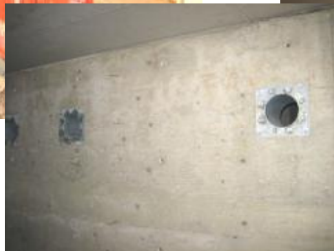
Img. 306, Img. 307. Detail of the holes in the walls for the ventilation system.
