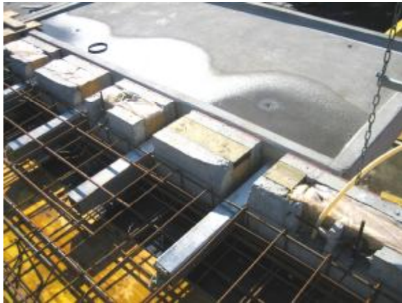
Img. 378. Metal parts of the balcony element, placed inside the cast concrete
