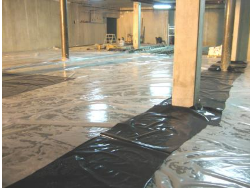
Img. 319. After the harden one of the concrete, it is covered with plastic to support the humidity and get the concrete well treated
