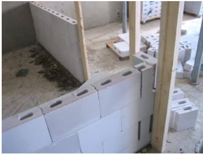
Img. 414. Assembly of a small format block wall and the wood opening frames
