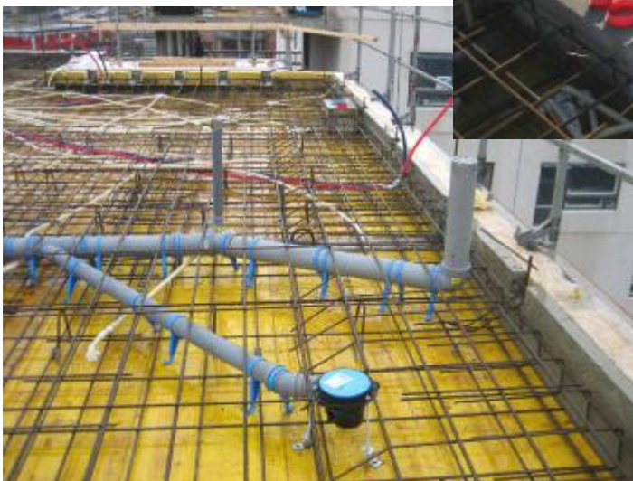
Img. 508 Facilities of drainage and the drain of a bathroom
