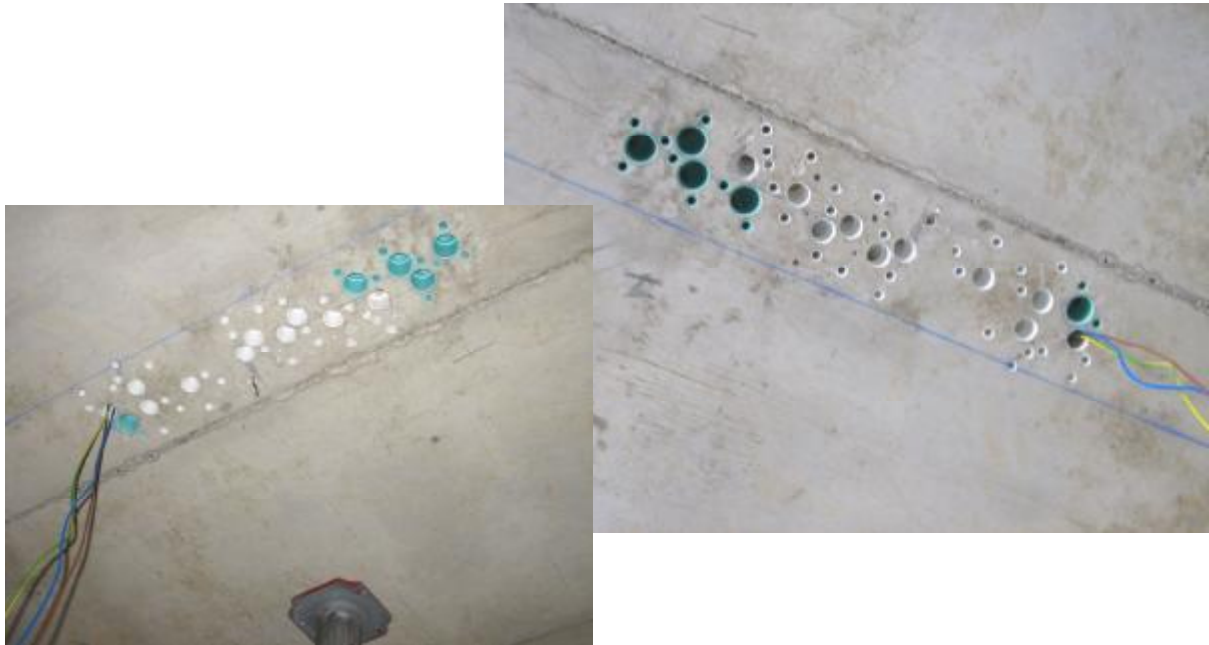
Img. 512, 513. Aspect of the full area of electrical installation pipes. These are above a partition wall where the pipes will continue
