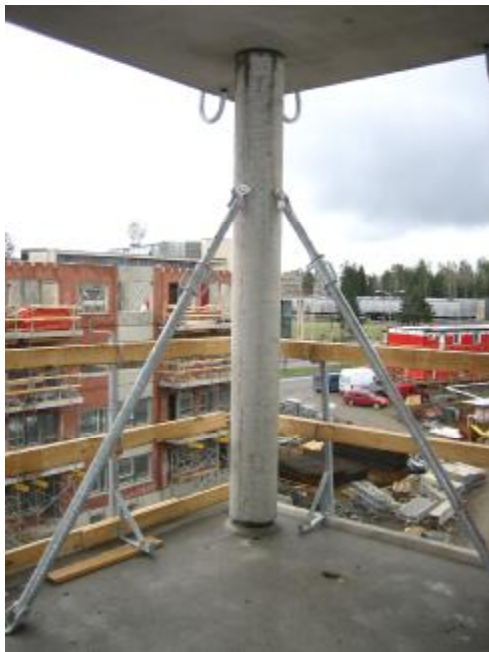
Img. 338. Column with with leaned supports
