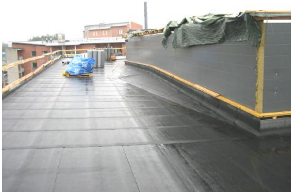
Img. 422. General view of the roof, after placing the first bituminous sheet
