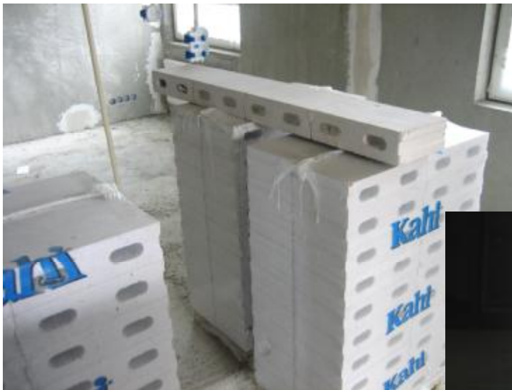
Img. 415. Stocks of blocks and piece lintel
