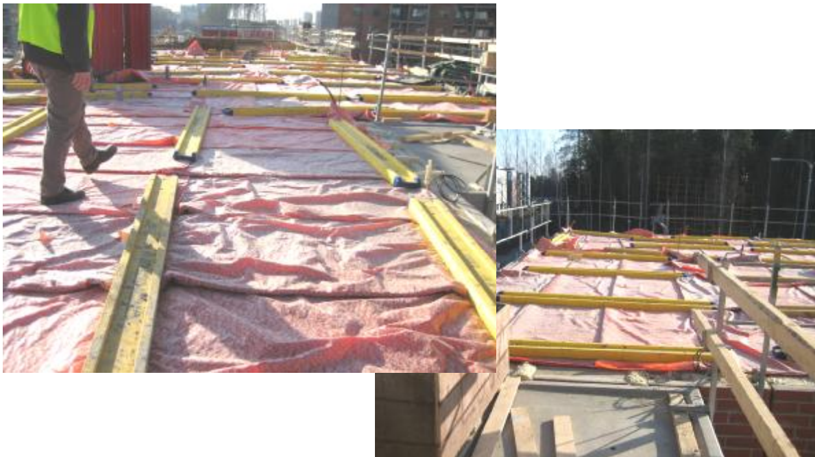
Img. 518, 519. Cast concrete slabs covered with blankets to keep the humidity and the heat
