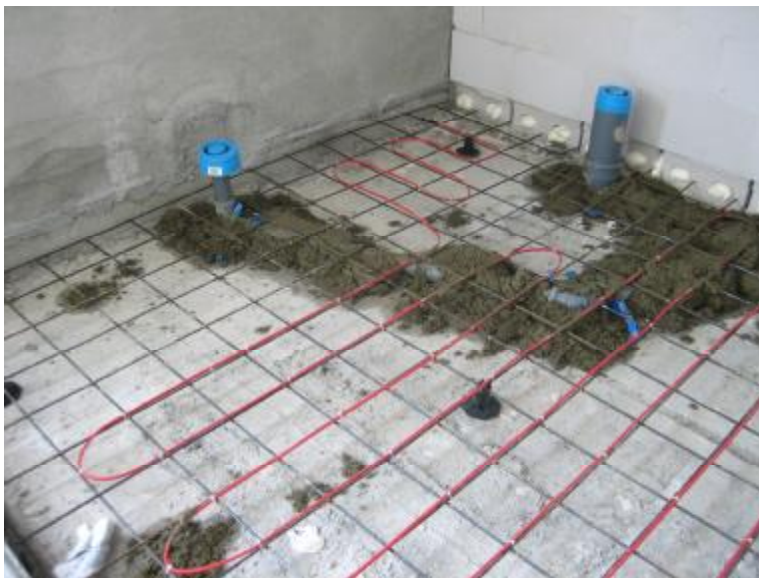
Img. 406, 408 Different sights of the floor electrical heating system
