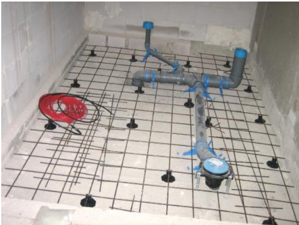
Img. 405. The bathroom areas are solved with thin slab elements that allow the placement of the drainage facilities on them
