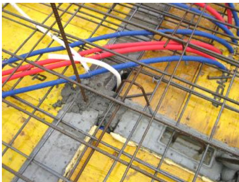
Img. 505. The top of some load bearing elemens that will be jointed with the cast concrete
