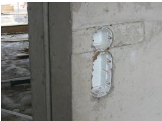
Img. 329. Boxes of the electrical installation included in the prefabricated panel
