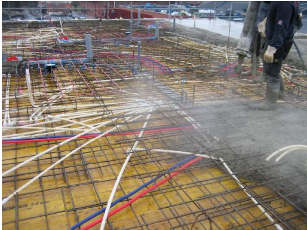
Img. 515. During the spread, the concrete detaches great quantity of steam, due to the hot temperature that it is
