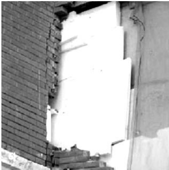
Figure 10. External masonry collapse.
