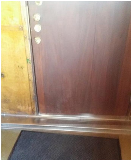
Image 18: Ferry door from the other side (Asp, 2016)
