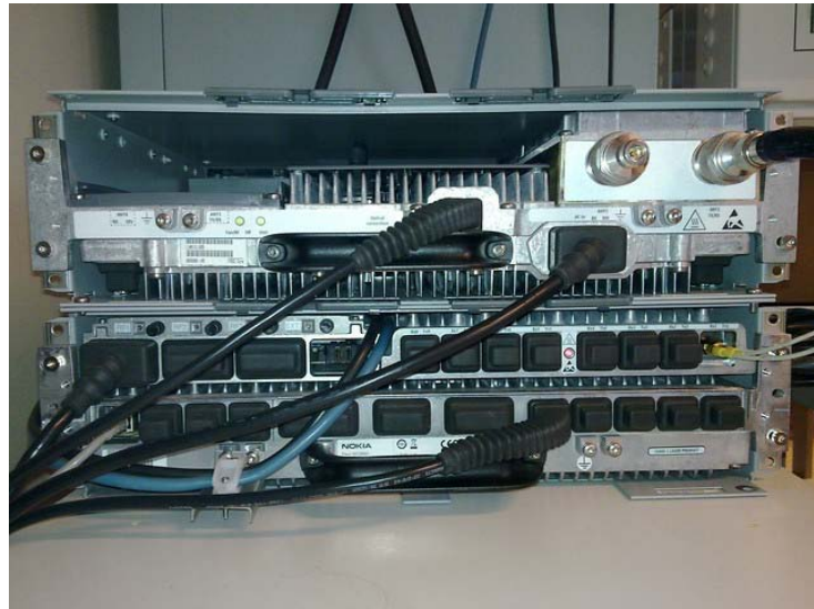
Figure 12. Nokia Flexi WCDMA Base Station
