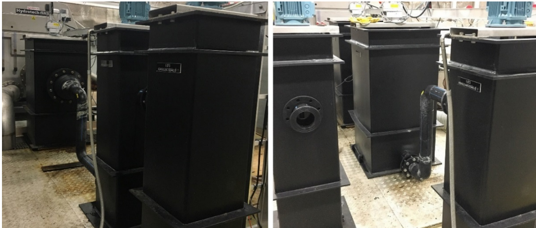
Figure 22. 2 coagulation and 1 flocculation basin (on the left), 1 coag. and 2 flocc. basins on the right
