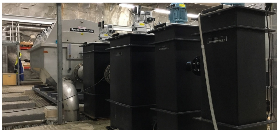
Figure 21. 2 coagulation and 2 flocculation basins
