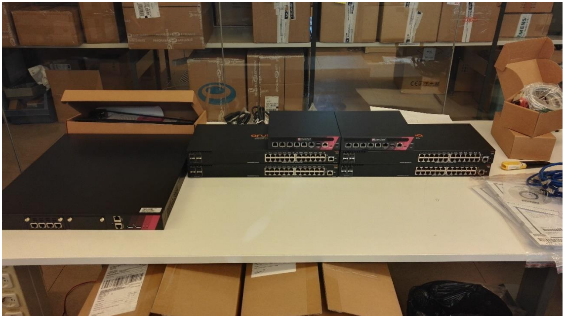
Picture 13. Setting up hardware
