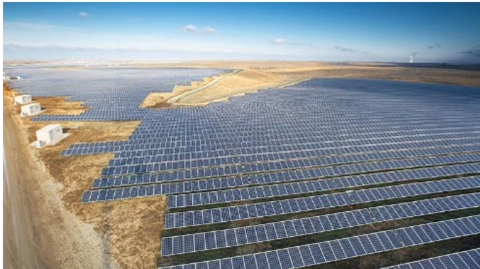
Figure 13. Solar panel power plant "Perovo" in the Crimea (LiveInternet 2015)
