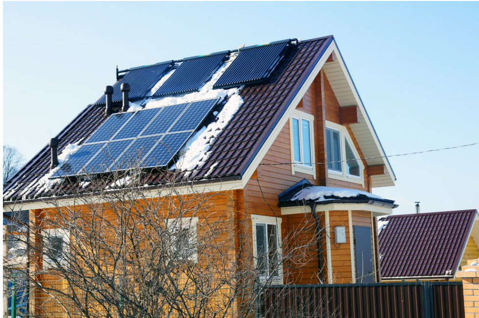
Figure 17. Solar panels on the roof (Ruba 2017)
