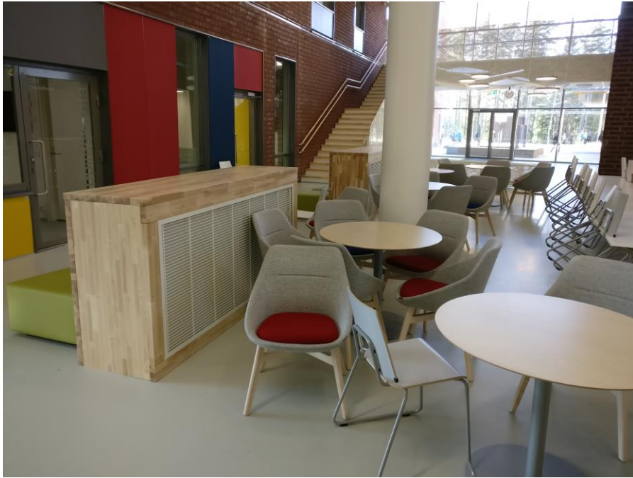
Figure 6.4. Lunch room. Supply air is distributed with integrated supply air diffusers
