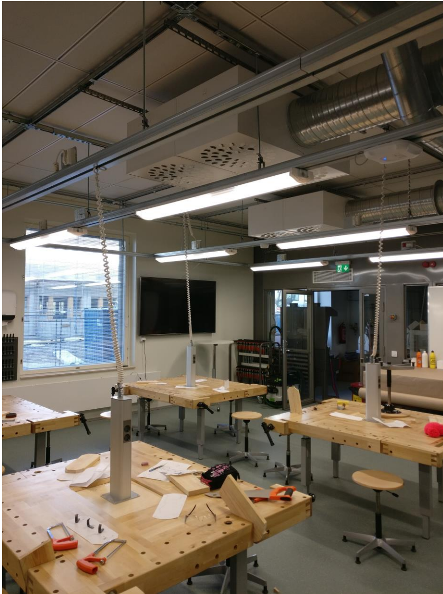
Figure 6.8. Technical work class room. Supply air is distributed with nozzle diffusers
