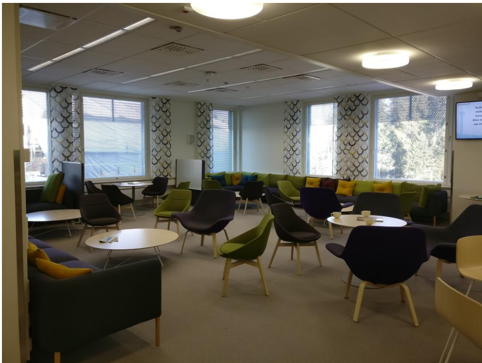
Figure 6.7. Teachers' recreation room. Supply air is distributed with nozzle diffusers
