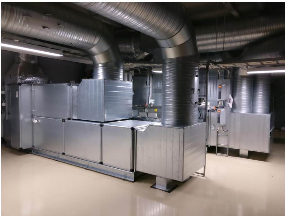
Figure 6.2. Air handling unit room
