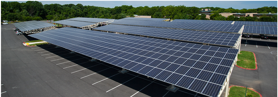
Figure 9. Solar panels installed in carport. Photo by- Matthew Borkoski
