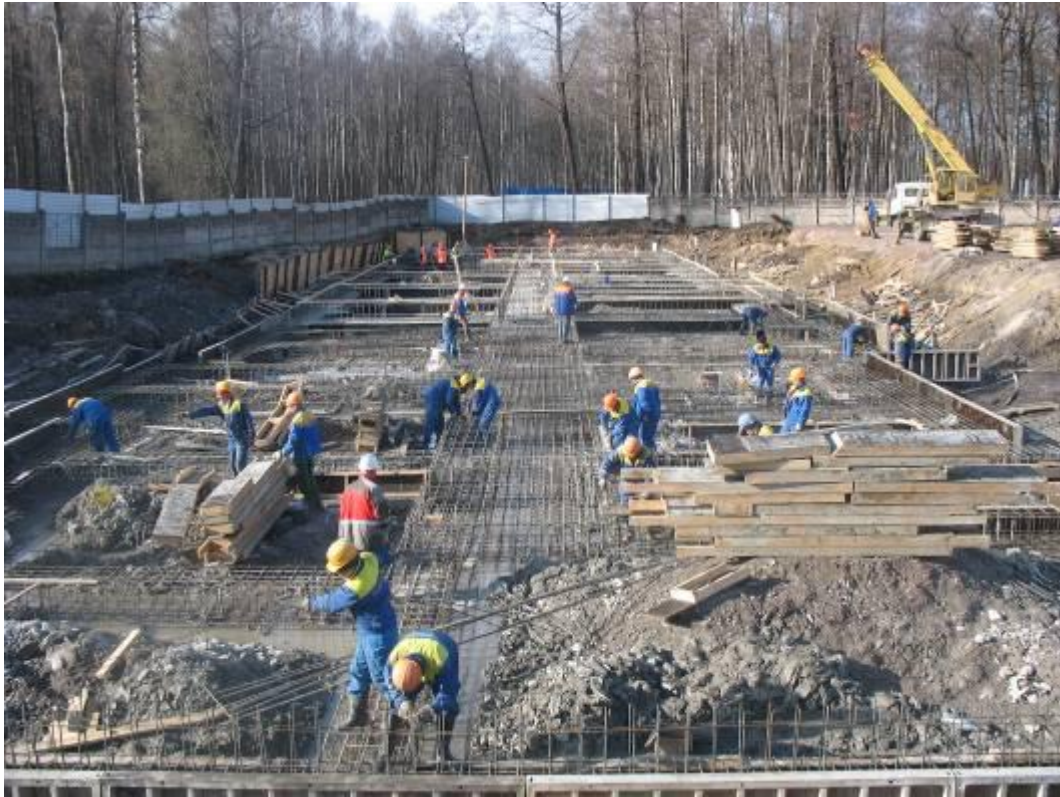
Figure 11. Absence of decks for walking above the reinforcement cage
