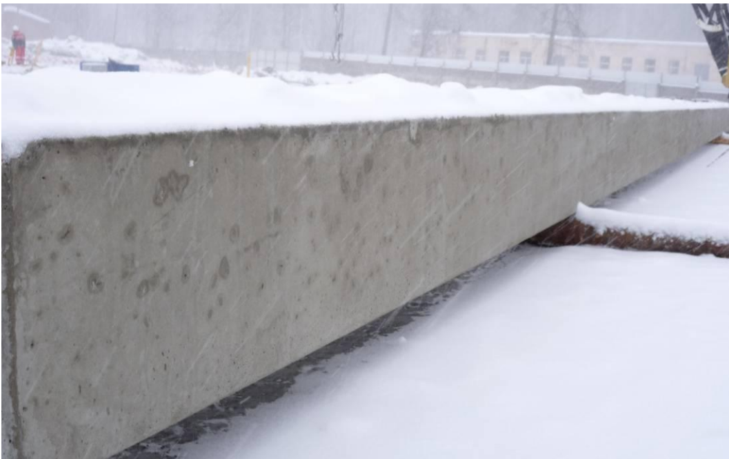
Photo 2. Defects of supplied piles
