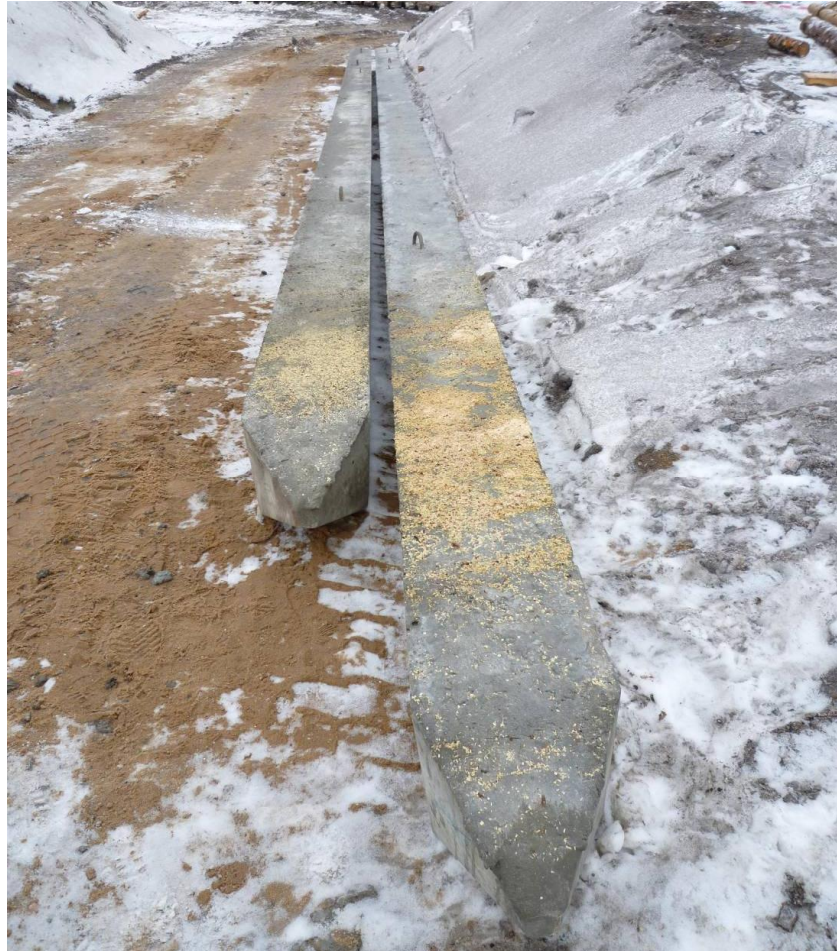
Figure 20. Defect of the pile length
