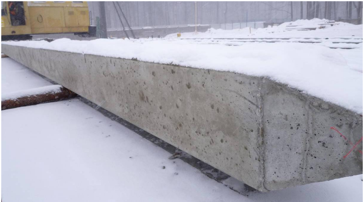
Figure 18. Pores and pile defects
