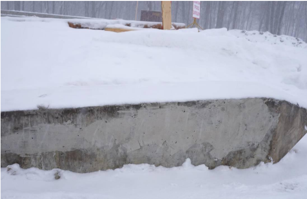
Photo 1. Defects of supplied piles
