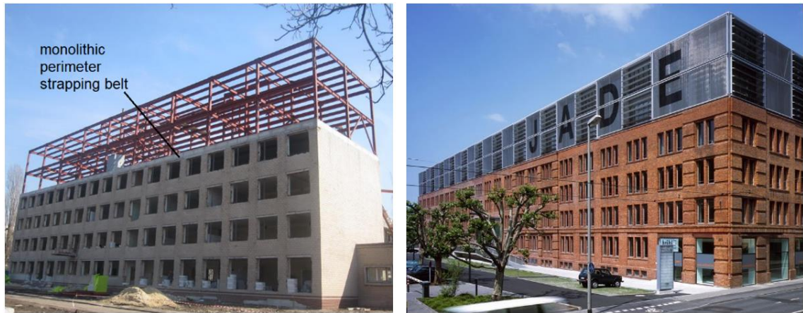
Figure 2. Examples of the refurbishment with two-storey superstructure placed on the old building masonry walls: reconstruction in Kiev (on left) (Metal Installation Service n.d.), office building in Frankfurt (Jo Franzke n.d.)
