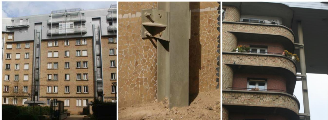
Figure 14. Roof extension using hot rolled profiles (Boulogne, Paris), details of the secondary structure junction, extra-column supporting the building extension (Caroli 2009).
