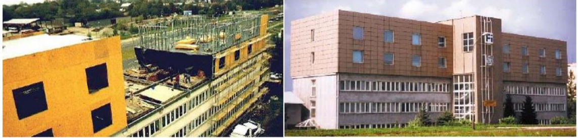
Figure 6. Vertical extension of the office building in Rzeszow (Poland) with steel use (Caroli, 2009)
