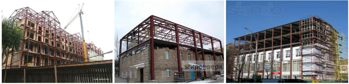
Figure 13. Examples of Flamingo superstructure performance: residential building in Minsk (Krasovskaya, 2013), frame made by Kronverk Metalwork Plant (n.d.) and storey-adding structure in Rostov-on-Don (Classifieds24. n.d.)
