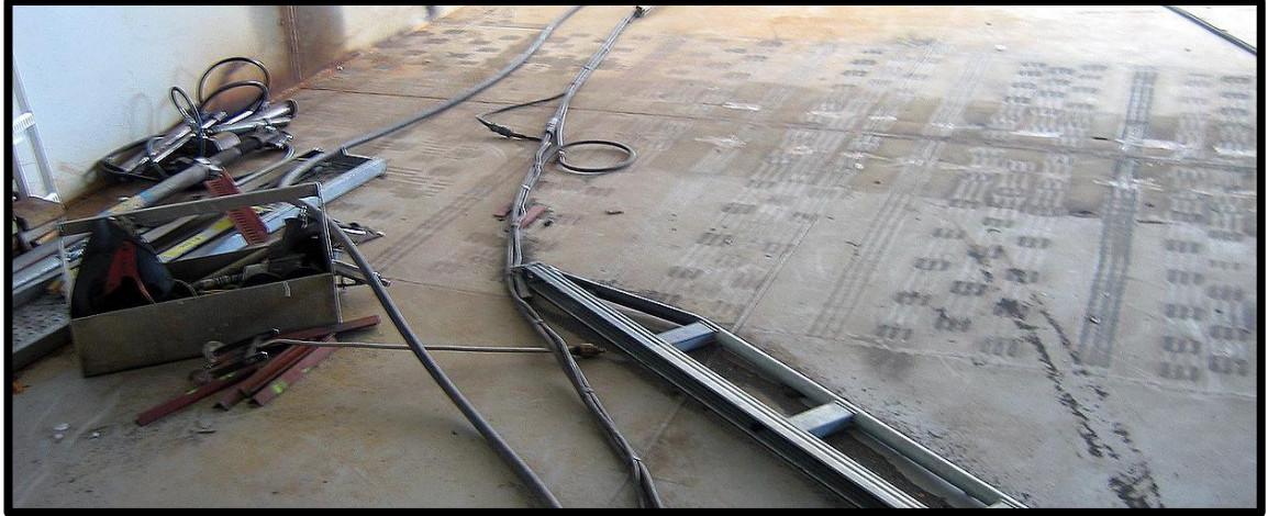
Figure 50 Additional cleaning required
