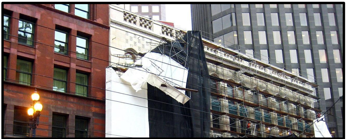
Figure 5 Scaffolding failure in San Francisco caused by stormy winds
