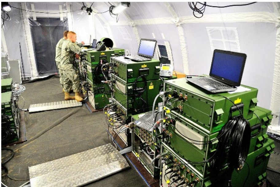
Figure 13: Operating Equipment Inside North Atlantic Treaty Organization Deployable Communication & Information System (Defense News, 2014)
