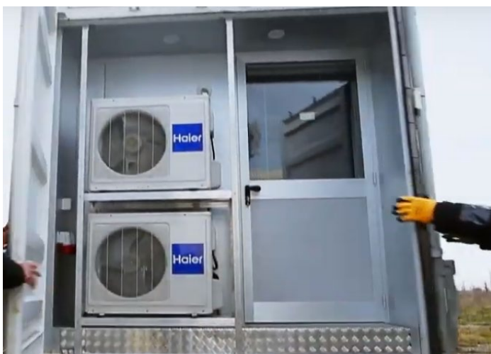
Figure 11: United Nations Modular Command Centre Air Conditioning Unit (United Nations Global Service Centre, 2017)
