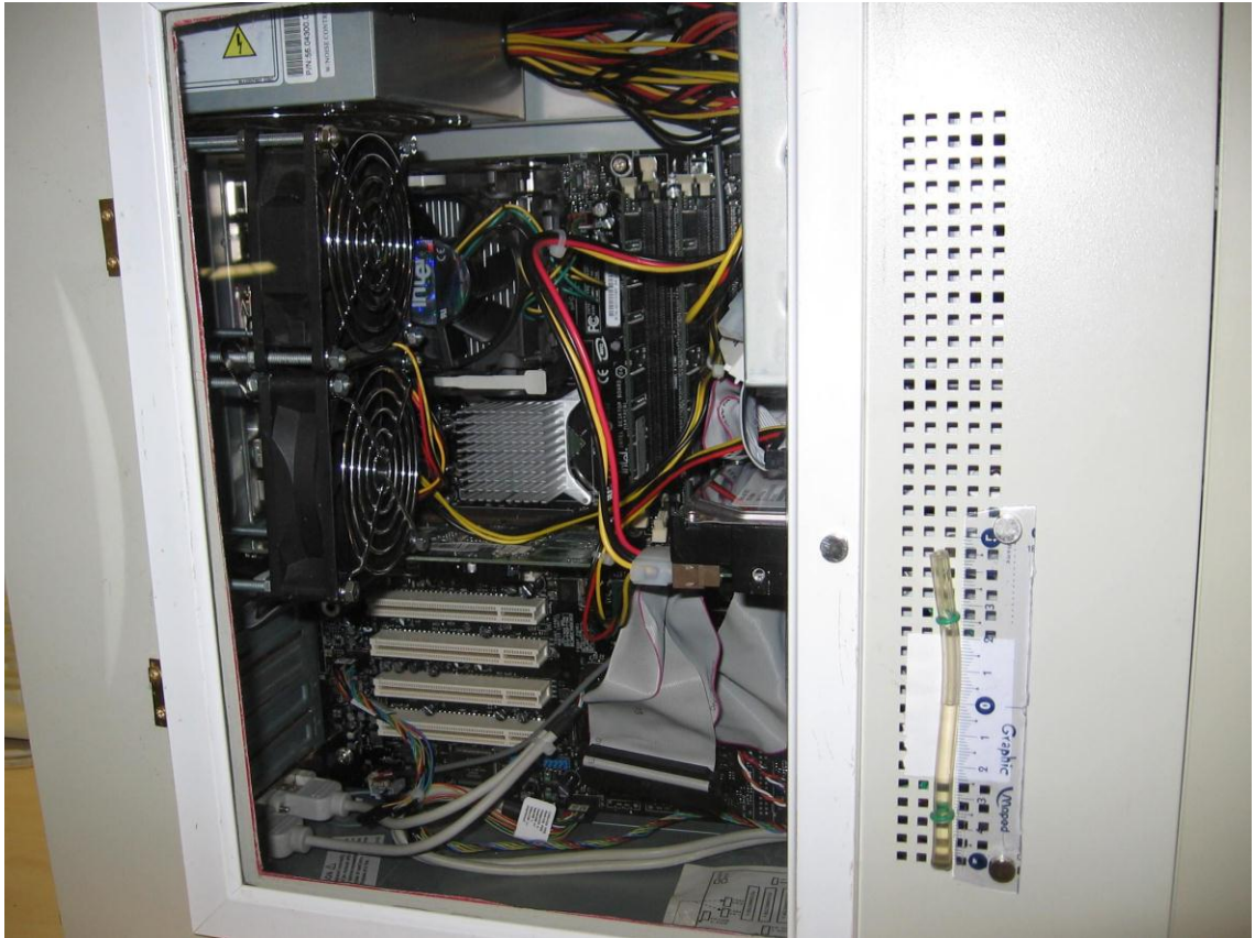
Figure 11: Fans inside the computer's case
