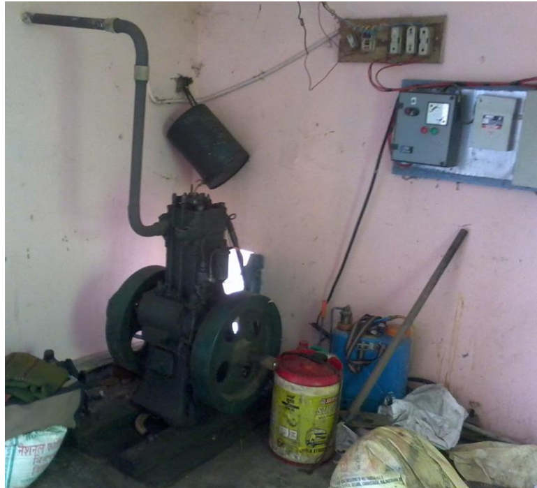
Figure 13: Electric pump run on diesel as a backup
