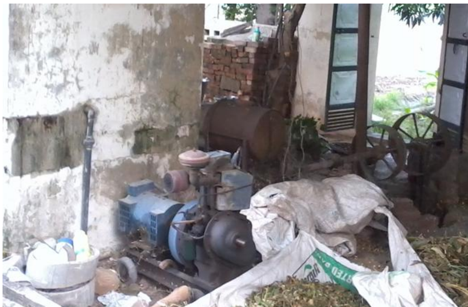
Figure 15: An electric pump motor run on solar energy
