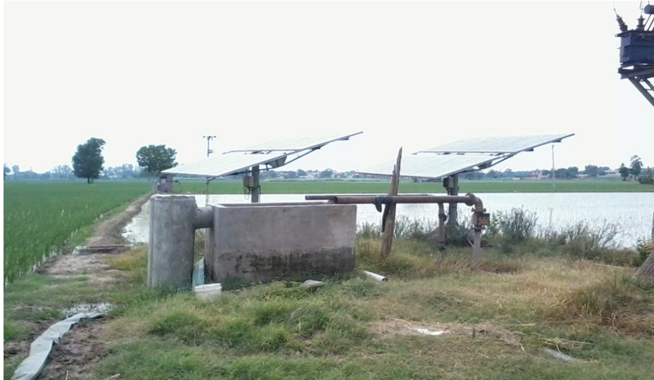
Figure 14: SWP in the field backed up by electricity
