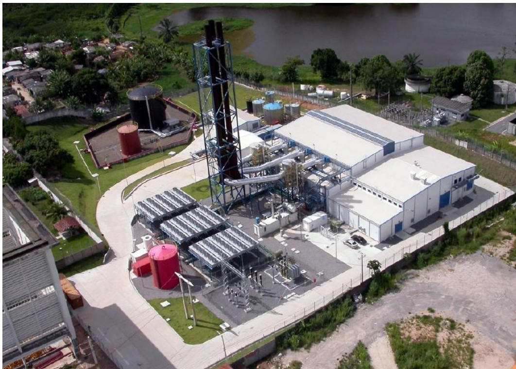
Figure 2. Ready Wärtsilä power plant in 2002 with three 18V46 engines. /29/
