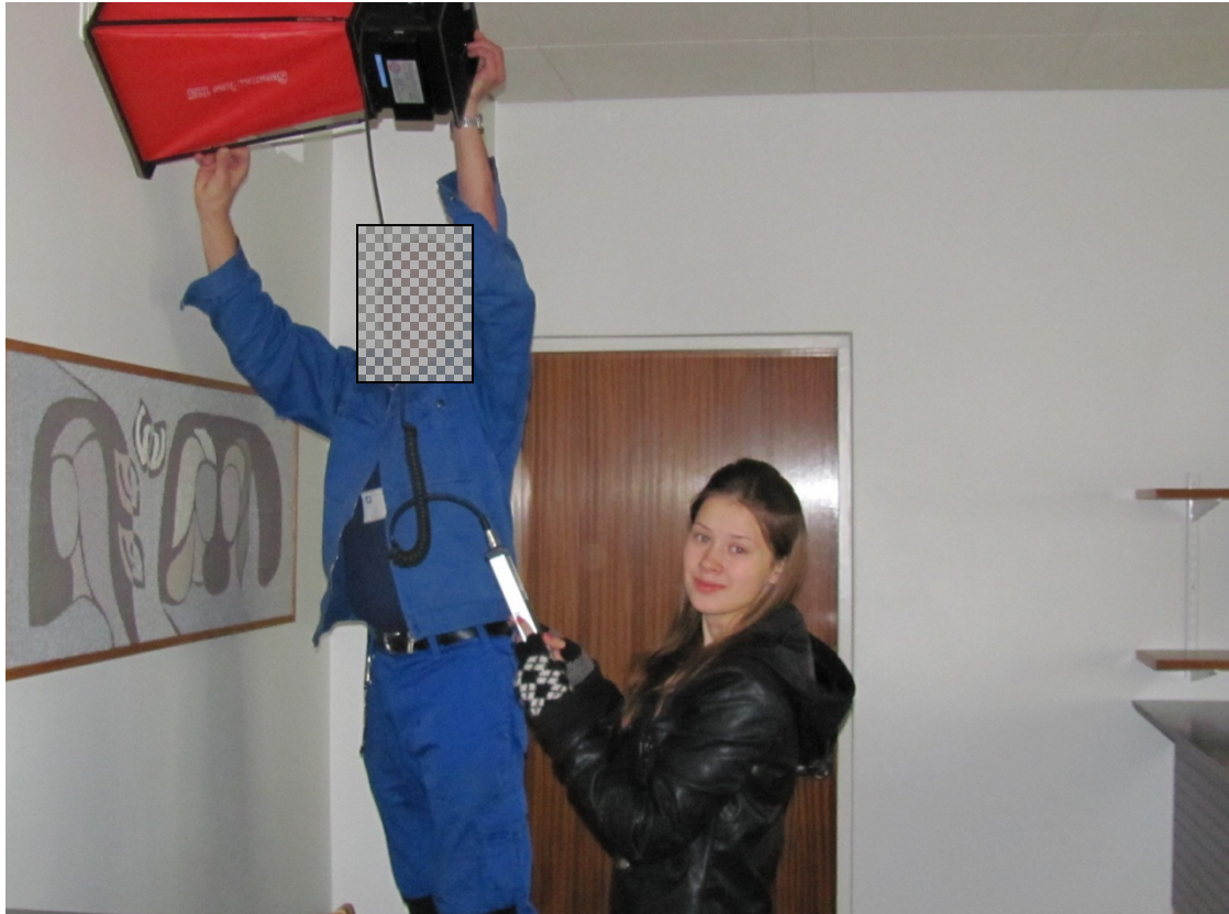
Figure 23. Air flow rate measurement in the room 1.
