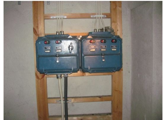
Figure 16. Fan on the attic.
