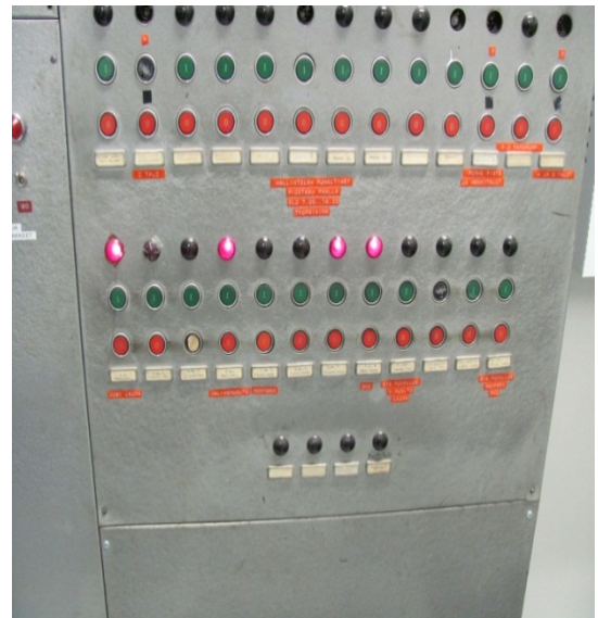
Figure 18. Distantly controlling system.
