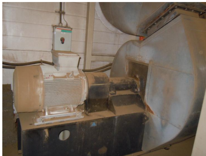
Figure 17 Flue gas fan in Karkkila
