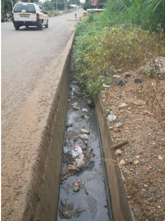
Figure 8. Gutters in the city area are usually littered.
