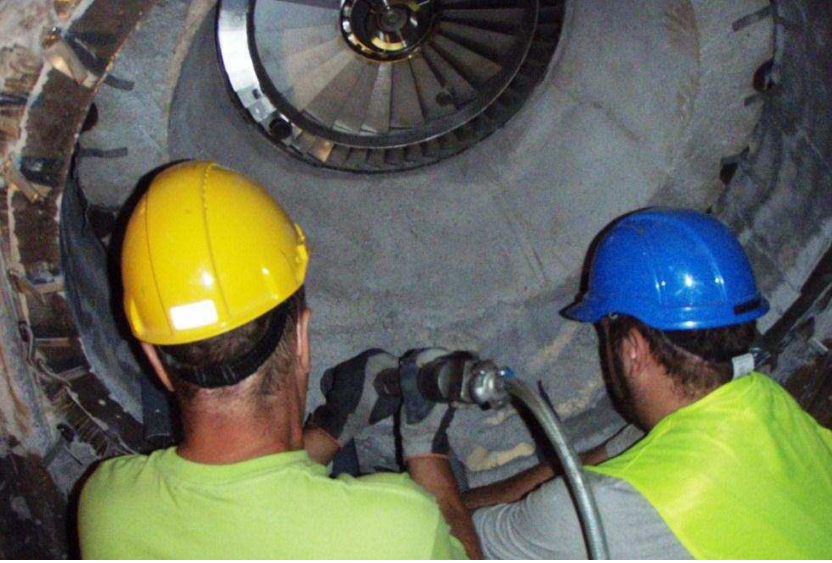
Figure 25. Refractory assembly, inside of the burner openings
