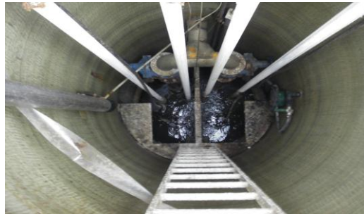
PICTURE 4.4 Glass fiber pump station in Lempäälä (Obijaju, 2011)
