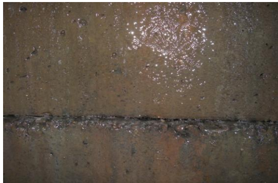
PICTURE5.1 Leaks from the walls and seams of the Manhole (Obijaju, 2011)
