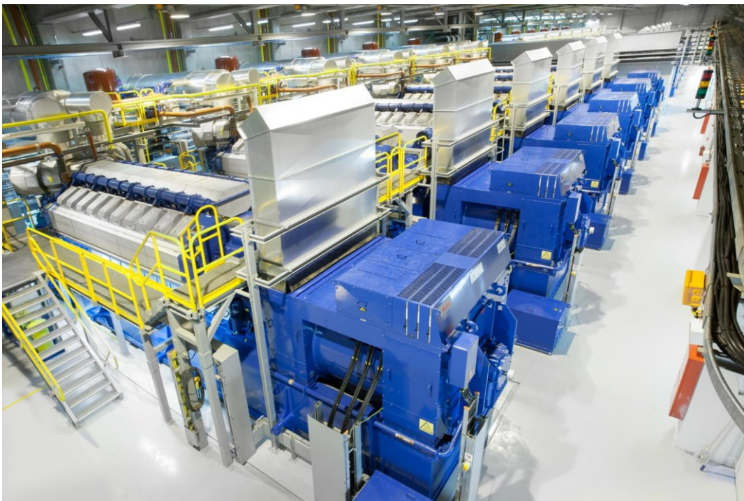
Figure 1. Engine hall inside Kiisa ERPP 1&2 Power Plant in Estonia (Image courtesy of Wärtsilä.) ©2021 Wärtsilä Corporation.
