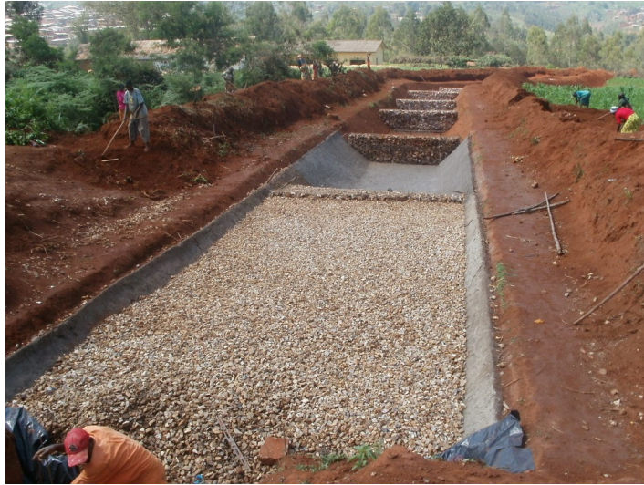
PICTURE 3. Construction of wetland (by Sustainable sanitation is licensed with CC BY 2.0.)
