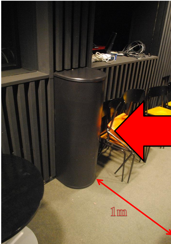
Figure 17. One of two semi-circular, wall-mounted diffusers Halton AFB in Mik-poli
