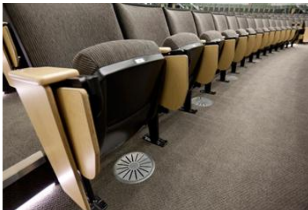
Figure 12.Supply air through floor diffusers with a twisting stream in the auditorium of the University of Amsterdam /4/
