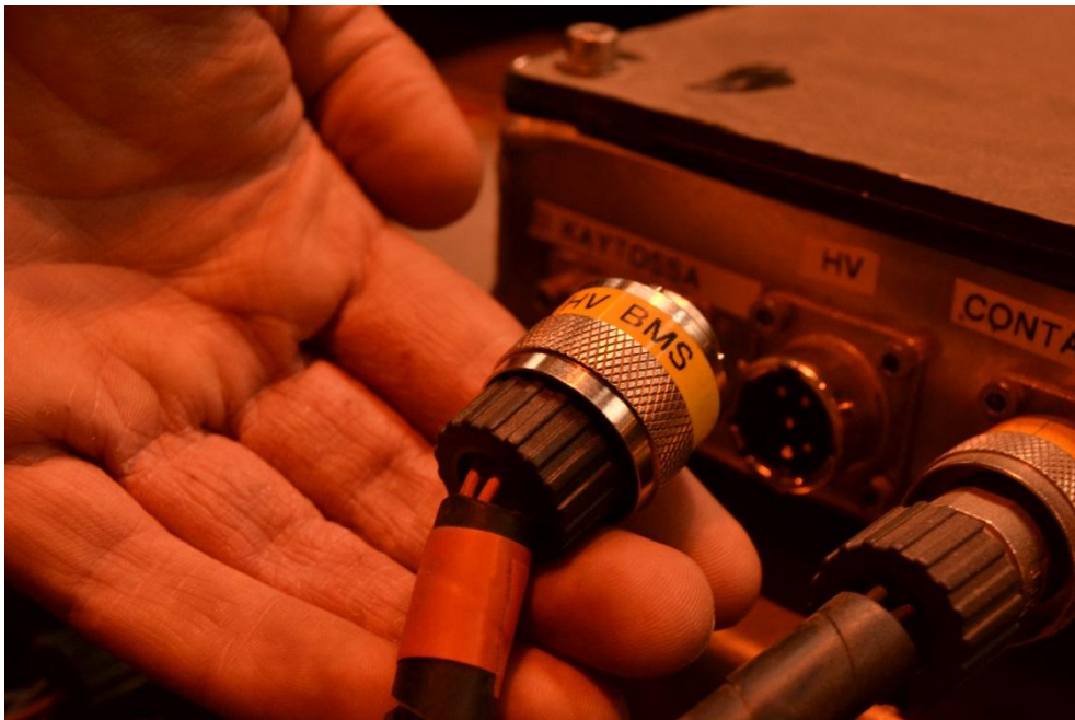
Figure 6. High voltage connections available in direct contact of hand in the old BMS -system.
