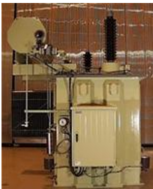
Figure 11. Neutral earthing reactor made by ABB /22/
