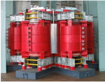
Figure 14. Superconducting FCL (35 kV/90 MVA) made in China
