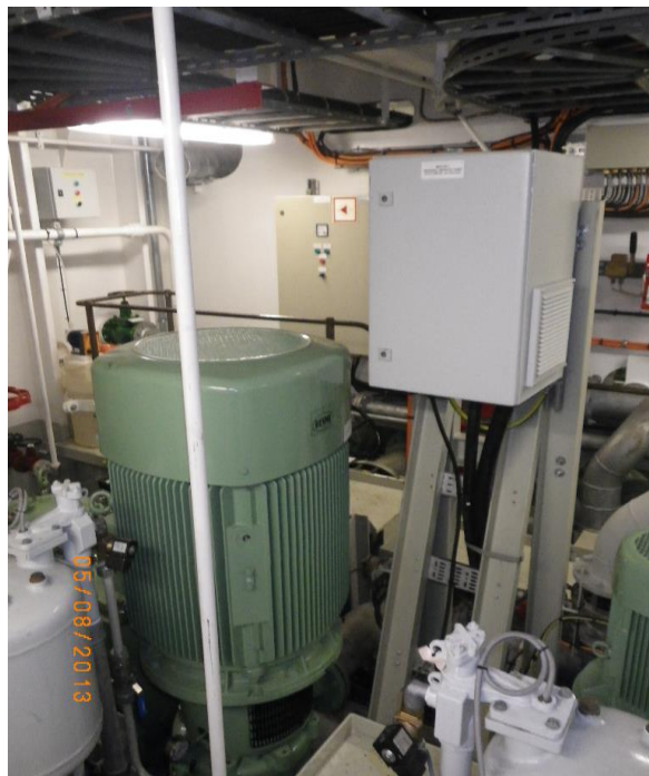
Figure 7. GS pump and soft starter
