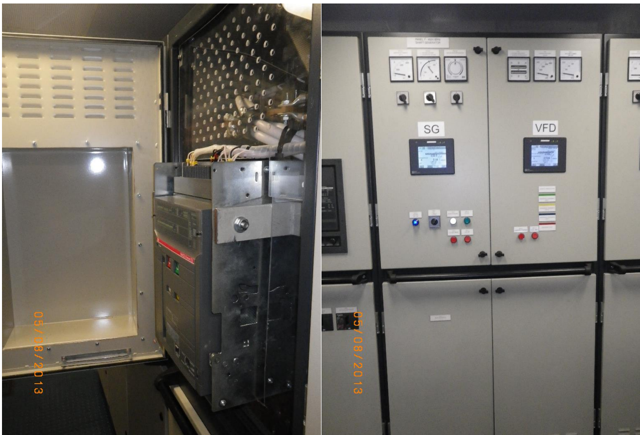
Figure 6. Retractable breaker and breaker control panel
