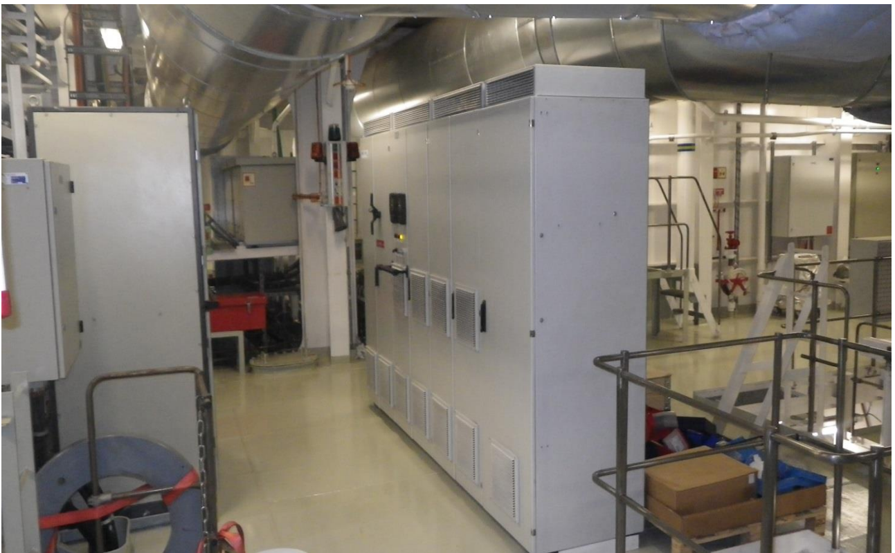
Figure 7. VFD unit cabinet.
