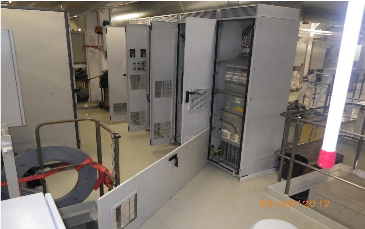
Figure 10. Temporary air flow aid to the VFD- unit.
