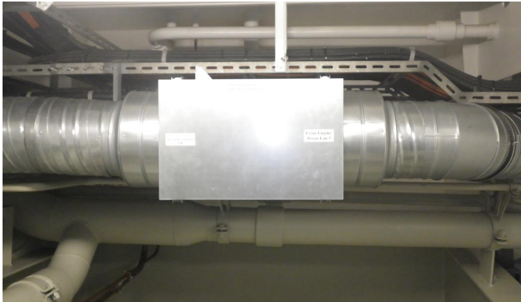
Figure 11. New cooling air filter.
