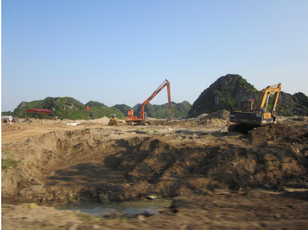
Picture 7. A view from the Cat Ba Amatina construction site (Photograph: Tatu Sundqvist 2011)
