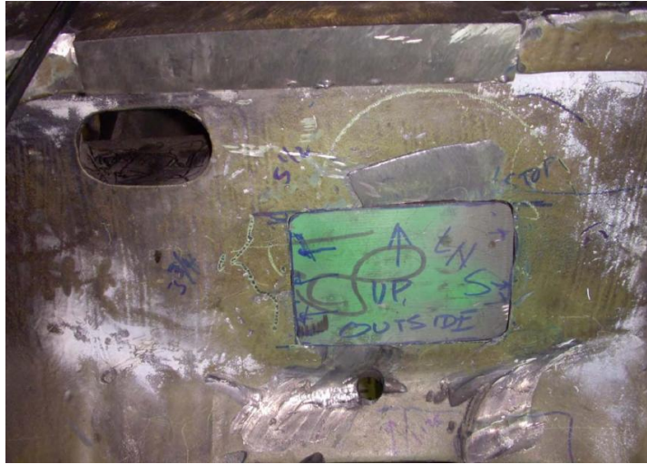
Figure 40. Damages with new patches stitched into place.
