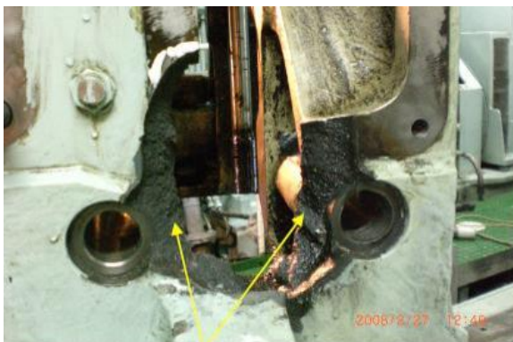
Figure 25. Cracked parts removed
